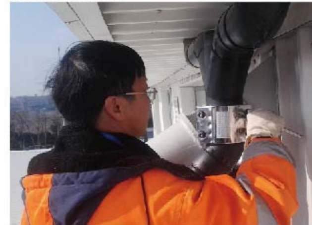
The welding joints of the siphon drainage pipeline break off. For secondary production, they adopt Zhuhong Repair Clamp.
