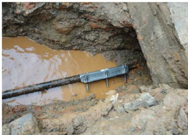
5. For the severely corrosive DN50 water supply pipe of Dalian Insulator Group, Zhuhong Repair Clamp repairs the leakage in very short time.
