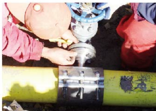
For DN150 pipe with DN20 branch, Daqing Oilfield adopts Zhuhong Multi-Function Tee Clamp to install with hoisting and sealing on nonstop pressured pipeline.
