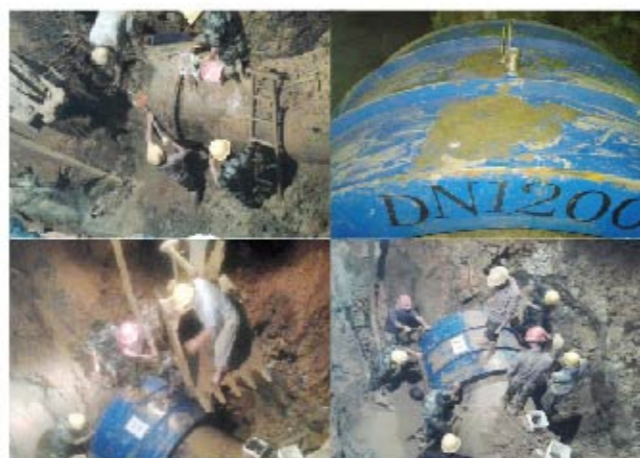
To Repair the socket part of DN1200 cement pipe burst in Hunan Water Group, they use Zhuhong Customized Non-Standard Socket Pipe Repair Clamp efficiently.
