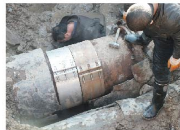
Shanxi Thermo-Power Corporation uses our DN500 Repair Clamp for their emergency repair of heating pipeline.
