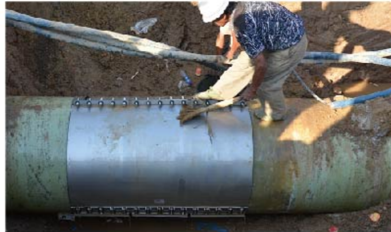
To repair the DN1200 GRP pipe of Hunnan Water Corporation conventionally, they have to stop the water pipe for more than 36 hours. However, using the Repair Clamp of Zhuhong instead just make it within 2 hours.
