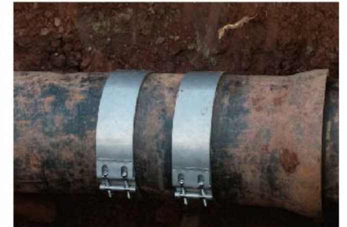
RCD Double-Section Short Clamps successfully connect the DN500 ductile iron pipeline buried in the ground.
