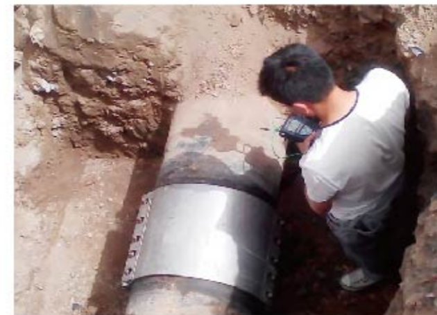
To solve the leakage of DN400 gas pipeline in Shanxi Huarun Gas Company, Zhuhong RCD Double-Section Repair Clamp performs quite excellent in fast repairing.
